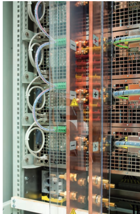
DC bus terminal
