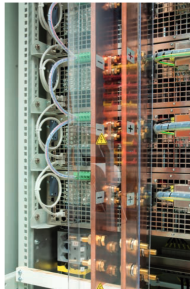
DC bus terminal
